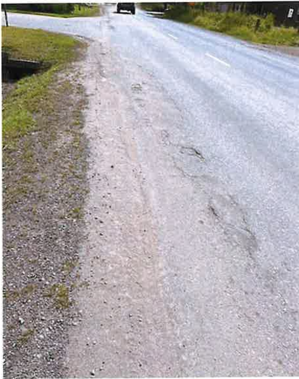
Condition of Davis Ave roadway surface looking south toward Blue Water Circle.
